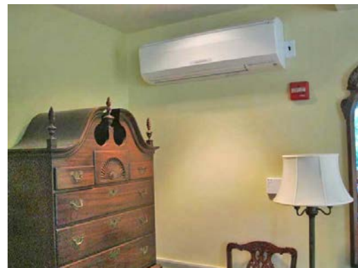
Mini-split on the wall brings heat and cold from the heat pump into the room.
