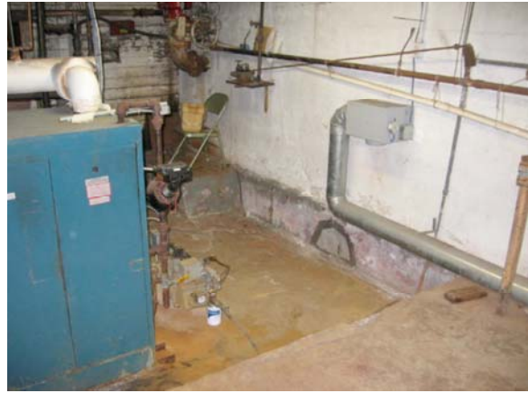
#3 — The atmospheric boiler required addition of fan-aided combustion make-up air, seen here wall mounted.
