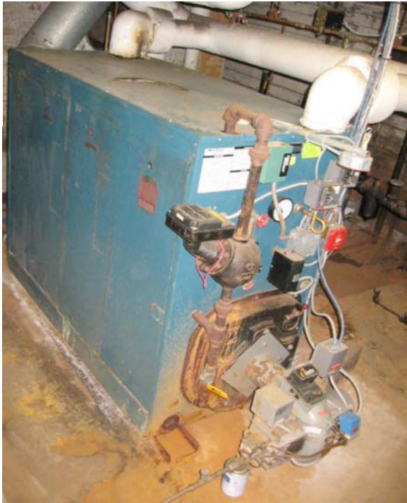
#1 — Oil-fired steam boiler was (efficiency 75%±) installed in 2001. Steam is less efficient given need to heat to 212° regardless of outside temperature. Steam is less readily zoned. Convert to higher efficiency solution, with geo-thermal an option, especially if AC is in the mix for future.
