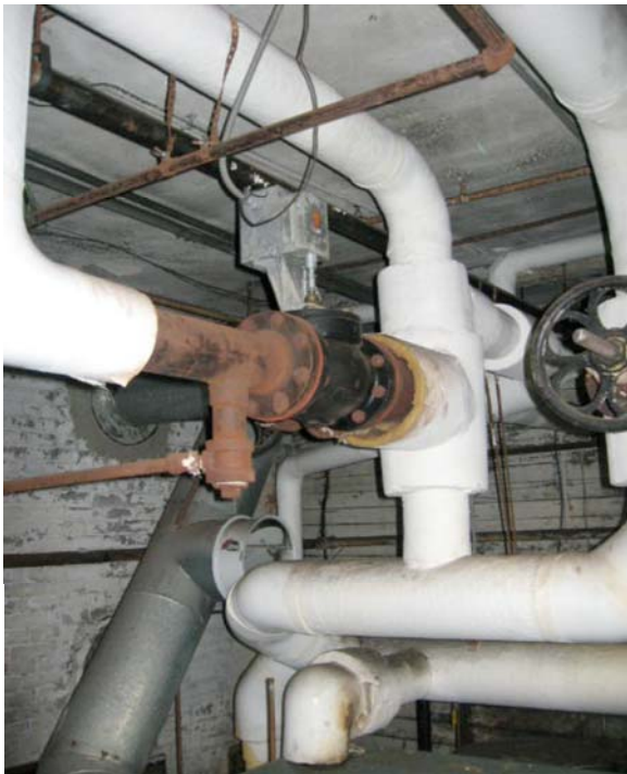
#2 — There are only two zones for heating, each with a valve controlled by in-space digital thermostats.
