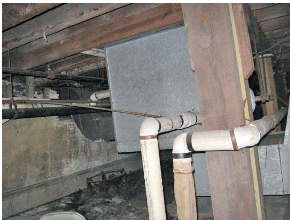
#6 — The radiator in the metal box is fed by the steam lines. Warm air moves upward, aided by cooler air returning through the duct system. The sanctuary can be converted to hydronic heating using in-floor radiation. Then insulate foundation and ceiling.
