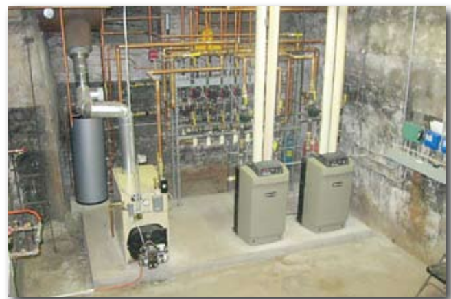
New Boilers at St. James Church.
